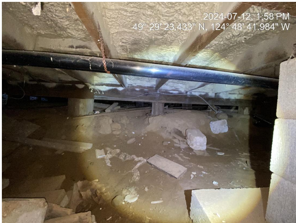
Figure 15 Wood rounds supporting floor beams set directly on the ground
