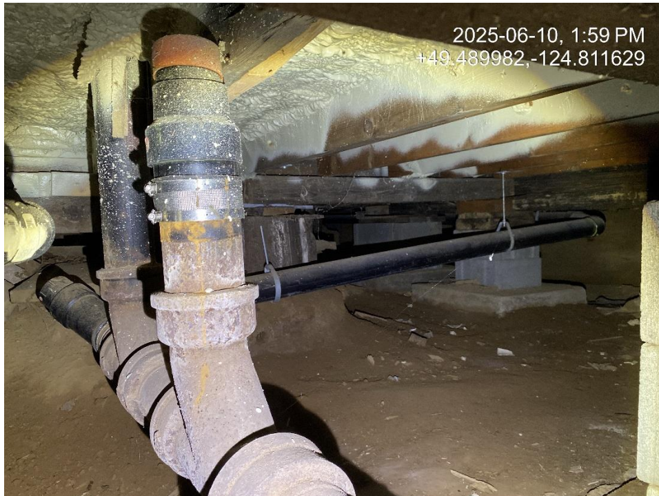
Figure 13 Wood and masonry supports
