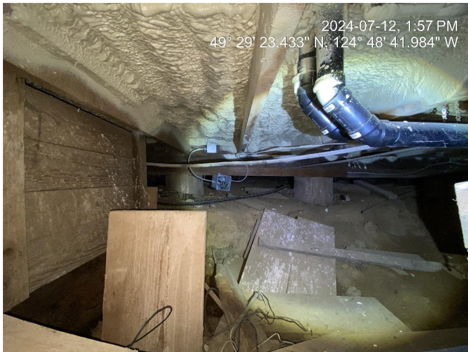
Figure 17 Wood rounds supporting floor beams set directly on the ground
